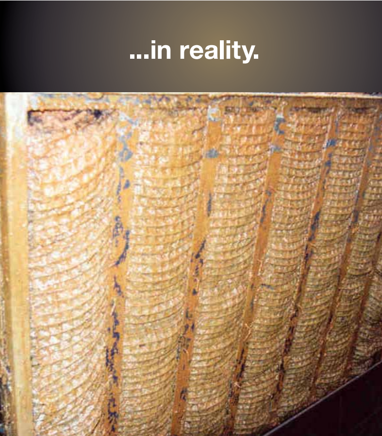
A Crutch to lean on because of a poorly designed primary coalescer.
